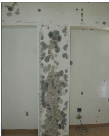
Mold growing on drywall
