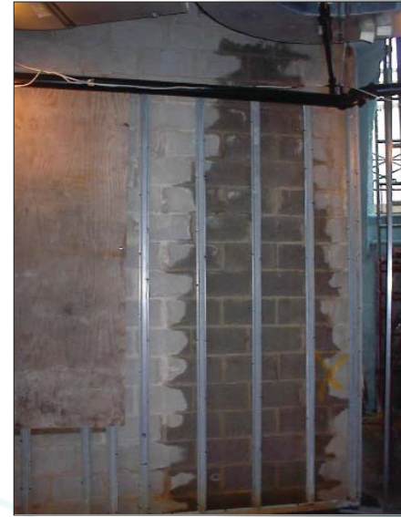
Mold developing on damp cinder-block wall
