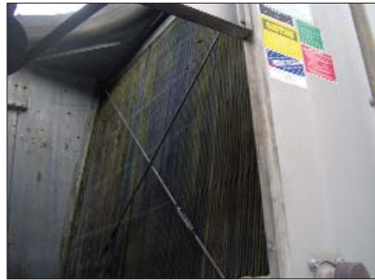
Algal Growth on Cooling Tower
