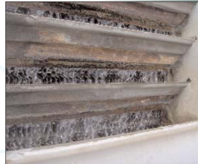
Bacterial Growth on Cooling Tower
